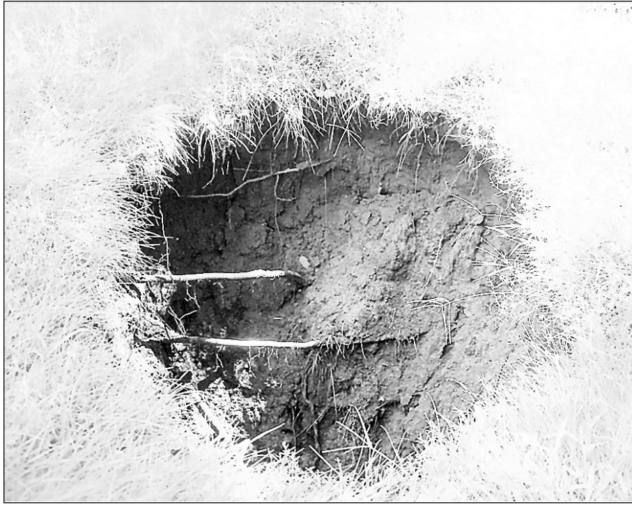
This eight-foot deep hole remains on the 500 block of Merchant Street in Gayville. The hole was created three weeks ago when part of a 70-year vitrified clay pipe collapsed because of heavy rain. The town is hoping to have the hole fixed within the next week.
