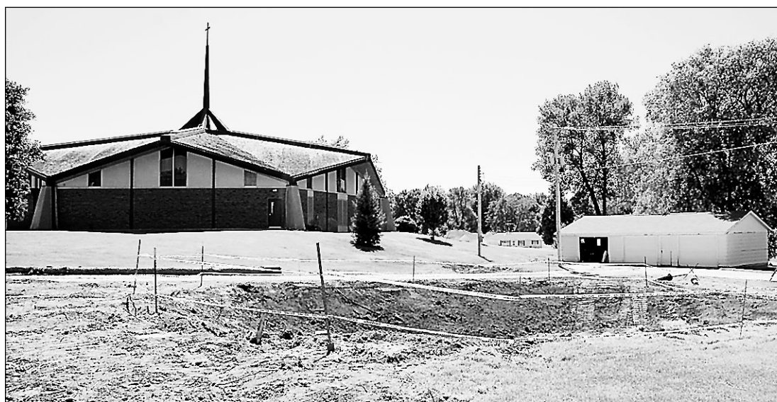
Caution tape surrounds the site where Hartington's Holy Trinity Rectory once stood. Built in 1913, the rectory was demolished last week after it was determined building a new facility would cost less than repairing the old one.
