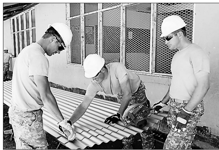
SDNG PHOTO: SPC. MANDA WALTERS Spc. Weston Blasius, (left) Spc. Waylon Blasius, (middle) and Sgt. Kirk Surat, measure and cut steel roofing material at the Pater van der Pluym School in Suriname's Brokopondo district. The Soldiers are all carpentry and masonry specialists assigned to the South Dakota Army National Guard's 155th Engineer Company from Wagner. Soldiers from the 155th are in Suriname as part of New Horizons 2011, a joint humanitarian mission between the Suriname government and the U.S. Southern Command with the goal of helping to improve the quality of life for the people of Suriname.
