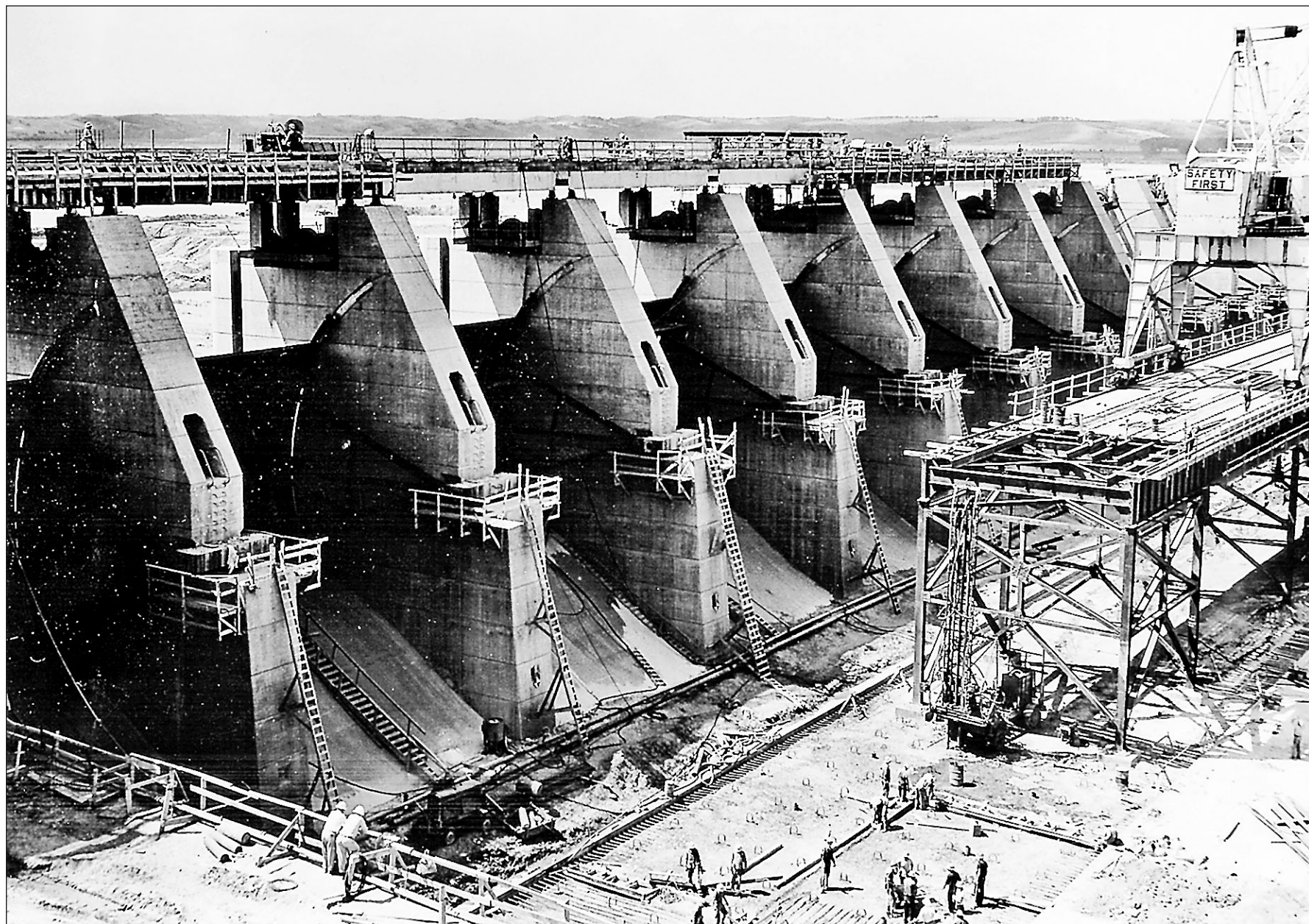
PHOTO: CORPS OF ENGINEERS ARCHIVES ABOVE: This image shows construction work being done on the Gavins Point Dam spillway bridge on May 16, 1955. The construction trestle on the right is being disassembled. TOP: A view of Gavins Point Dam in July 2011, with the spillway discharging a record 160,000 cubic feet per second due to the historic flooding on the Missouri River.
