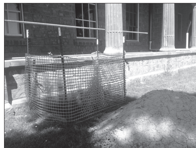
PHOTO COURTESY OF DAKOTA TERRITORIAL MUSEUM The exterior of the Mead Building has been getting ready for the installation of new sewer and water. The front of the building has a few large holes exposing portions of the foundation for ease of access. There should be water access to the building before winter, which will help the efficiency of the interior plaster work. The connection of important utilities will also help to make the building much more comfortable for our workers as we continue the restoration. If you have questions about the project or events please contact us at the Dakota Territorial Museum at 610 Summit Street (in Westside Park), on Facebook, visit our website at www.meadbuilding.org , or call us at 605-665-3898. The museum is open 10 a.m.-5 p.m. Monday-Friday and noon-4 p.m. weekends.
