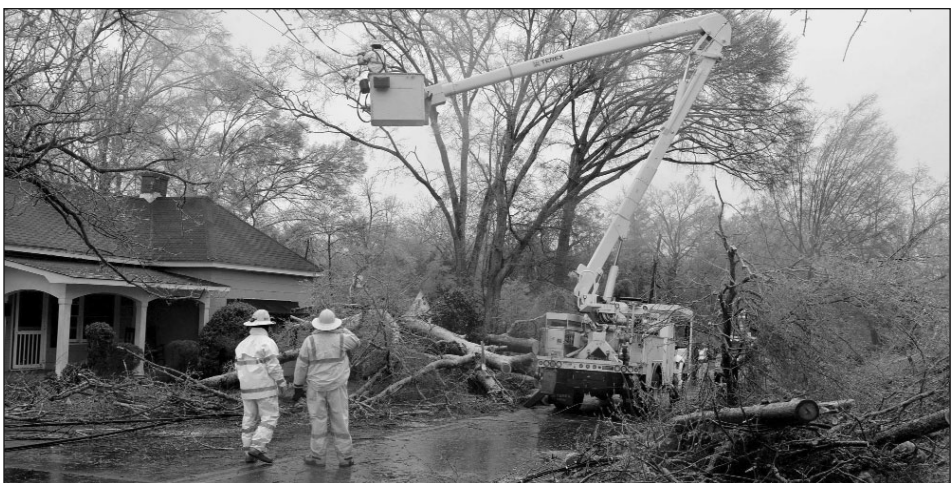
KENT D. JOHNSON/ATLANTA JOURNAL-CONSTITUTION/MCT Griffin Power employees work on downed power lines during the winter storm on Maple Drive in Griffin, Ga., on Wednesday.
