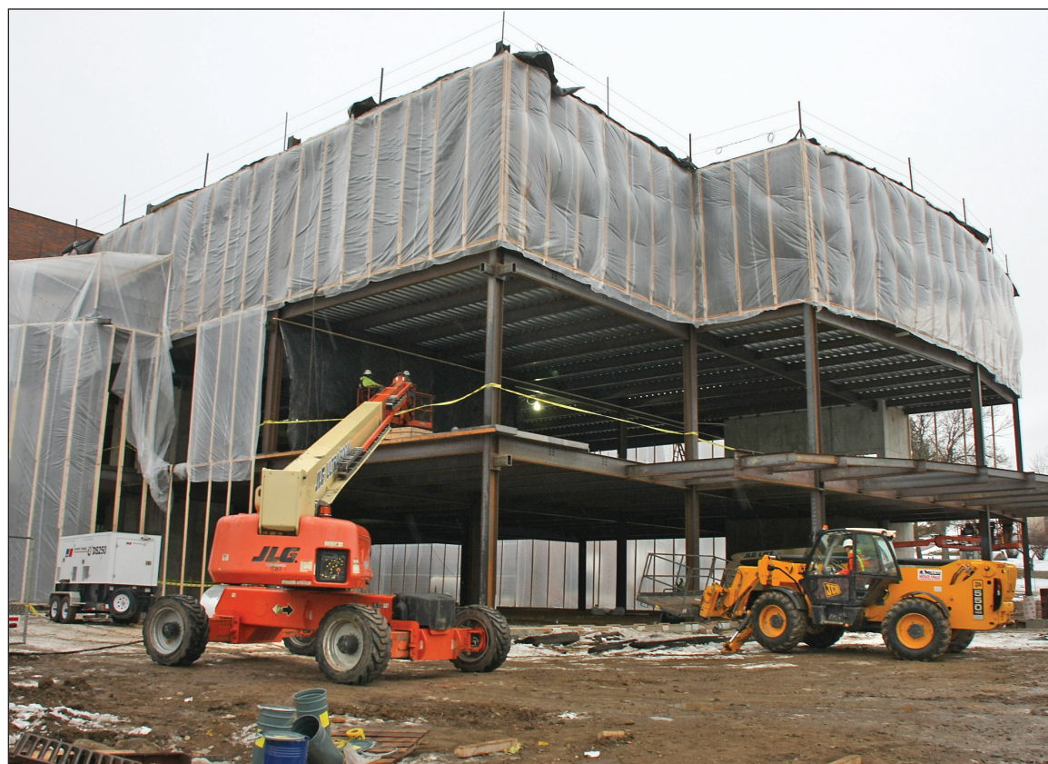
KELLY HERTZ/P&D Work continues to progress on the $11.7 million Northern Lights addition at Avera Sacred Heart Hospital. It was by far the largest project to get a building permit from the City of Yankton in 2012.
