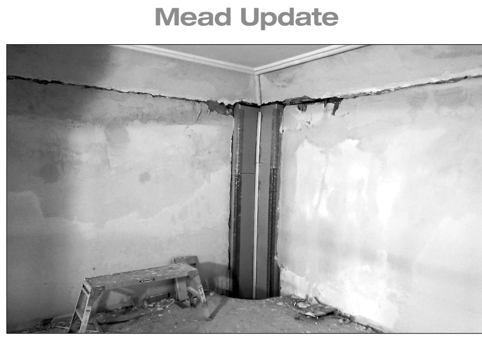
PHOTO: DAKOTA TERRITORIAL MUSEUM Pictured here is some of the reconstruction happening in the foyer over the marble staircase as part of the plaster restoration project. Roger Huntley and Gregg Homstad report that the northern corners of the foyer are near complete. Moulding repair is coming along well and the only areas left to replace are in the south corners. When all the plaster is fixed in the foyer, the crew will be able to move onto the painting stage of the foyer. Things are busy at the museum as we prepare for collections care training in February. On Feb. 13, Crystal Nelson will be conducting basic collections care training for new volunteers, area museum patrons and anyone interested in learning. Feb. 23-27, conservator Terri Schindel will be conducting more advanced training and working with people in a hands-on setting. The training sessions are possible thanks to the IMLS grant the museum received. If you are interested in helping prepare the collection for moving, please contact the Dakota Territorial Museum. If you have questions about the project or events you can contact us at the Dakota Territorial Museum at 610 Summit Street (in Westside Park), on Facebook, or call us at 605-665-3898. The museum is open noon-4 p.m. seven days a week.
