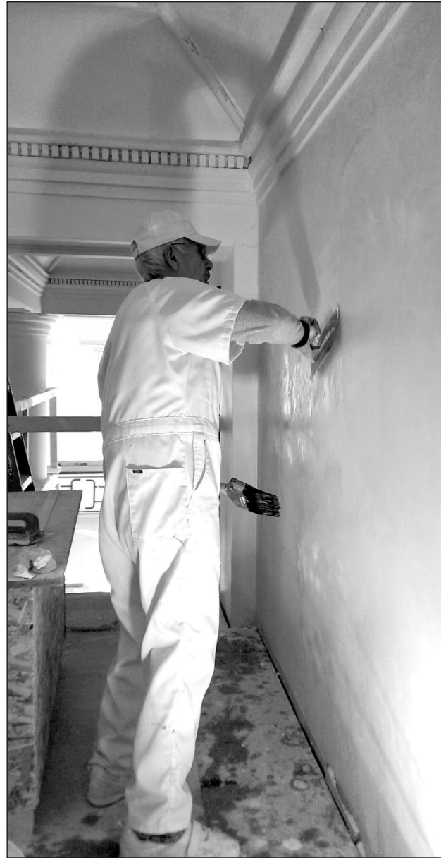
PHOTO: DAKOTA TERRITORIAL MUSEUM Shown here, the plastering in the high foyer area is nearing completion at the Mead Building. Roger Huntley, shown bringing the plaster surface to a shine, has been donating his time and expertise to work with project director Gregg Homstad since December. The intent is to finish plaster and paint work above the main staircase so that the scaffolding can be removed as soon as possible. If you are interested in volunteering at the museum, we have an important training day coming up. On Feb. 13, Crystal Nelson will be conducting basic collections care training for new volunteers, area museum patrons, and anyone interested in learning. Feb. 23-27, conservator Terri Schindel will be conducting more advanced training and working with people in a hands-on setting. The training sessions are possible thanks to the IMLS grant the museum received. If you have questions about the project or events you can contact us at the Dakota Territorial Museum at 610 Summit Street (in Westside Park), on Facebook, or call us at 605-665-3898. The museum is open noon-4 p.m. seven days a week.
