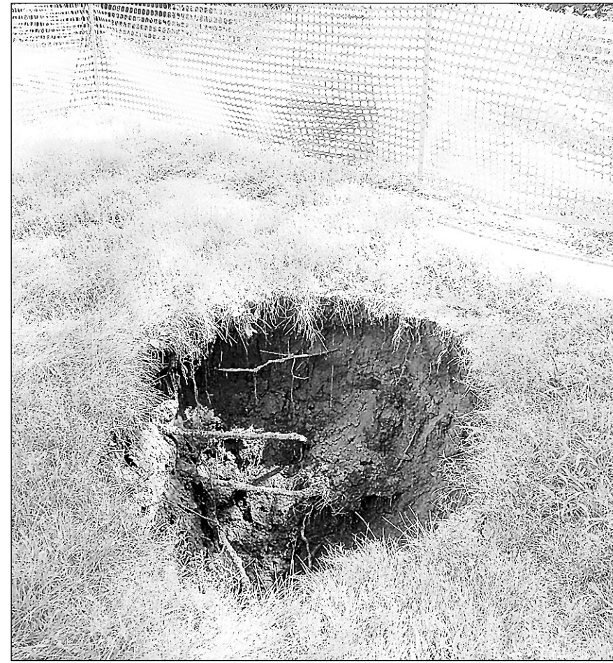
TRAVIS GULBRANDSON/P&D A collapsed drainage pipe in Gayville is causing concerns about the safety of areas above the 1,500 foot clay pipe that was built more than 70 years ago. City residents are waiting on a possible loan to replace the aging pipe, but for now people who live near the 8-10 foot deep by four and half foot across hole are wondering if it is safe to be in their yards.
