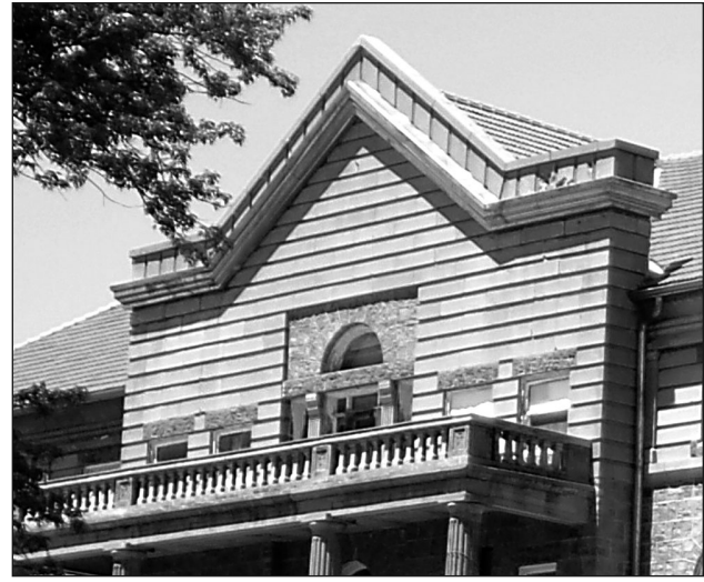
PHOTO: DAKOTA TERRITORIAL MUSEUM Work will soon begin on the decorative parapet wall above the third floor balcony. Modern techniques will be used to remedy the historical problems that have plagued the structure in this area. Passersby will be able to see the work being done, but when completed the repairs will not be noticeable. Don't forget to participate in our Mead Magnet contest. When you see a magnet of the Mead Building around Yankton and Yankton County, take a picture and post it to our Facebook page (give us its location) and be entered into a drawing for $50 — drawings held at the end of July and August. Check out www.meadbuilding.org . Here you can make monetary donations to the project. If you have questions or would like more information about the project, please contact the Dakota Territorial Museum at 610 Summit Street (in Westside Park), on Facebook, or call us at 605-665-3898.
