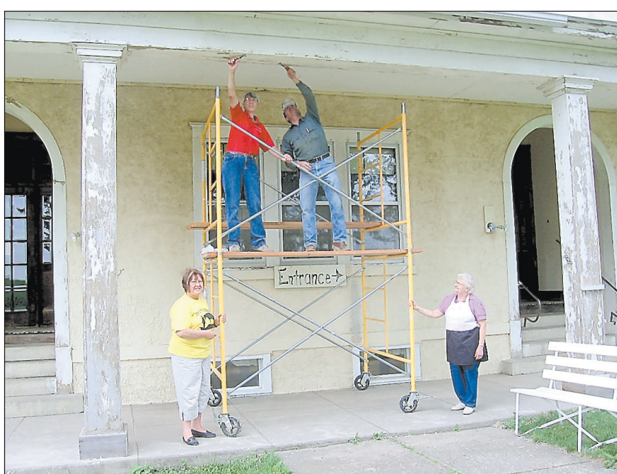
PHOTO: LINDA WUEBBEN Laborers work to scrape a portion of the old St. Philip & James Catholic School building near St. James, Neb. The building has been purchased by the St. James Marketplace and will be converted into a meeting place.
