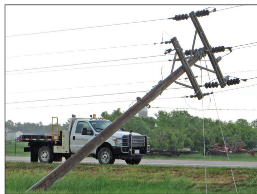
This power pole near the intersection of Highway 50 and West City Limits Road was pushed over by strong winds during a storm that moved through Yankton at mid-afternoon Saturday. Power outages at several businesses and residences were reported.
