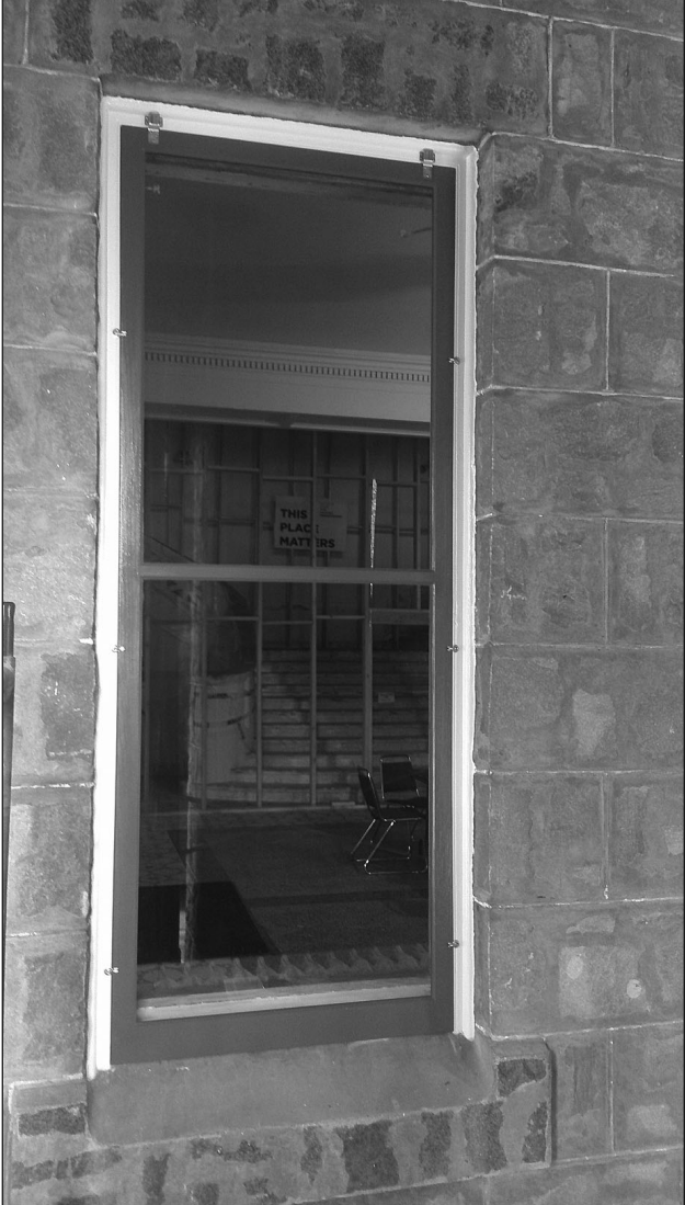
PHOTO COURTESY OF DAKOTA TERRITORIAL MUSEUM Alas, the first newly constructed storm windows have been complete and install (pictured above). The work of the Mead Building crew and Chalkstone Woodworking continues to be a real asset to the project despite Mother Nature's soggy and ever changing weather conditions. Don't forget to participate in our Mead Magnet contest. When you see a magnet of the Mead Building around Yankton and Yankton County, take a picture and post it to our Facebook page (give us its location) and be entered into a drawing for $50 - drawings held at the end of June, July, and August. Check out www.meadbuilding.org . Here you can make monetary donations to the project. If you have questions or would like more information about the project, please contact the Dakota Territorial Museum at 610 Summit Street (in Westside Park), on Facebook, or call us at 605-665-3898.
