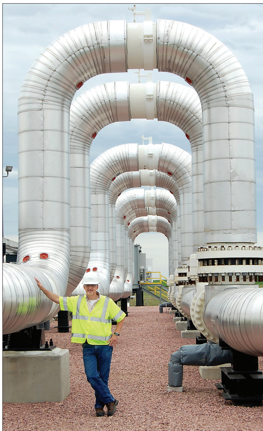
RANDY DOCKENDORF/P&D TransCanada spokesman Rob Latimer stands Thursday amidst a portion of the Keystone pump station near Hartington, Neb. TransCanada officials offered a tour and explanation of the pipeline operation for American Indian tribal members and Cedar County, Neb., officials.
