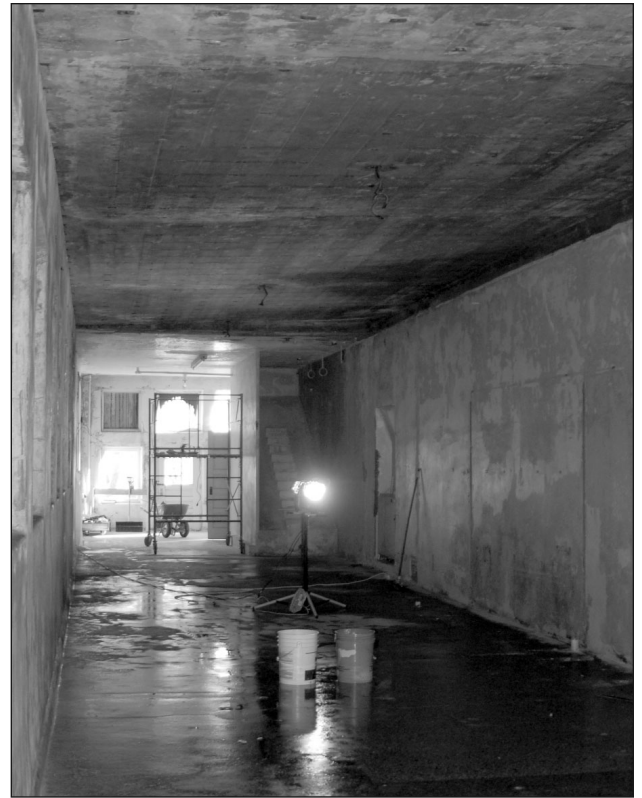
PHOTO: DAKOTA TERRITORIAL MUSEUM With winter trying to move into Yankton, the work crew at the Mead Building has been busy trying to fill gaps and cover windows missing glass. So far, the weather hasn't stopped the work inside the building. Demolition of the center hallway bathrooms is done and workers are focusing on wall demolition on the first floor west wing. Committee members are working to create a Mead Building Project website to help keep everyone updated on progress. On this website you will be able to make contributions, see work completed and take a virtual tour of the building. If you like youtube.com, there are several clips about the Mead Project available to see. If you have questions about the Mead Project or the museum, please stop by and see us at the Dakota Territorial Museum, 610 Summit Street (in Westside Park) or like us on Facebook. Museum hours are noon-4 p.m. seven days a week.
