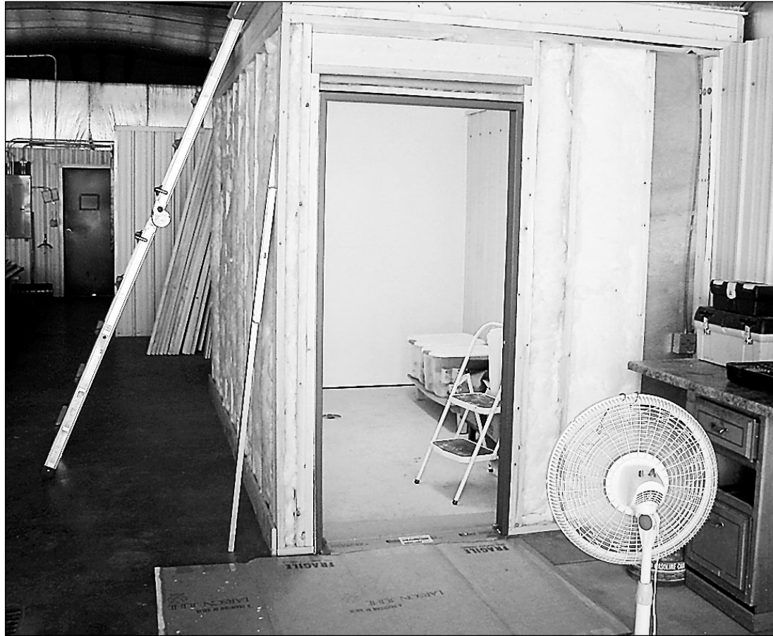
Construction on Volin's resource room continues. The room needs some steel on the sides and some trimming. The room will hold Gayville-Volin's food pantry, an LCD projector and a laptop when it's completed.
