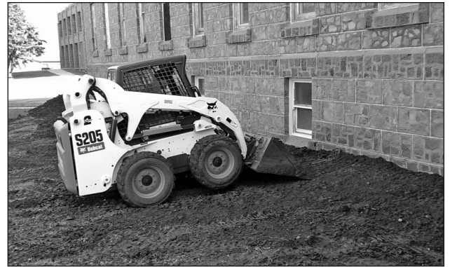
PHOTO: DAKOTA TERRITORIAL MUSEUM Dirt work around the Mead Building has been completed. The added dirt will help flow the water away from the building, eliminating the water entering the basement. A special thank you to Dr. Brad Kleinsasser for helping move the dirt with his Bobcat. There is still time to sign up for the Historic Preservation Class being held through RTEC. The classes will focus on plaster work and will be held at the Mead Building. For more information, contact the museum or look for the poster on our Facebook page, or call RTEC at 605-668-3482. The deadline is Oct. 1. Check out www.meadbuilding.org for the latest updates and check out our new blog on the website. If you have questions or would like more information about the project, you can contact us at the Dakota Territorial Museum at 610 Summit Street (in Westside Park), on Facebook, or call us at 605-665-3898.
