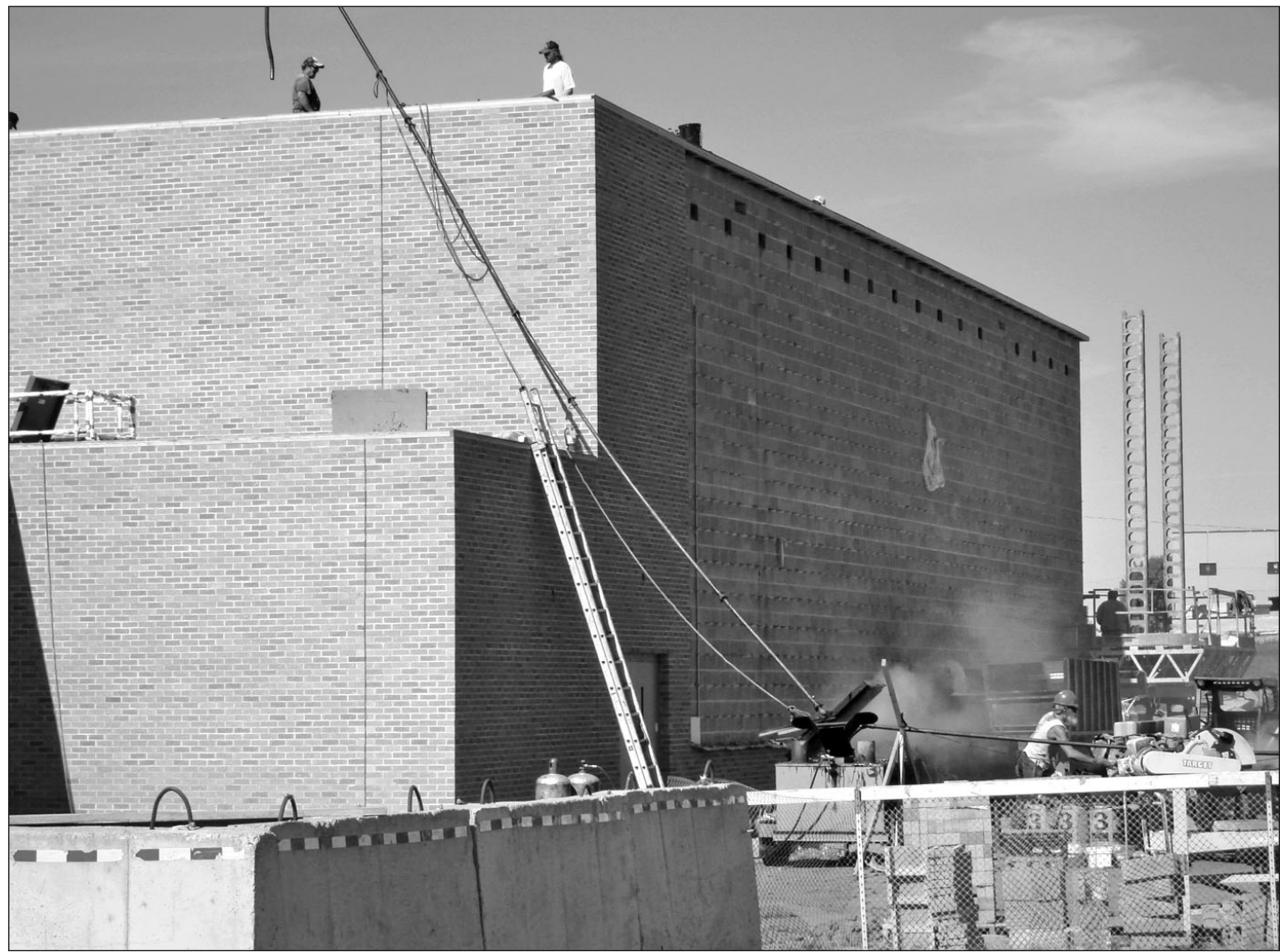
This 2009 photo shows the construction work on the new addition at Stewart Elementary School. The addition, which was opened in 2010, added a new gym, a library, a computer lab and two special education rooms.
